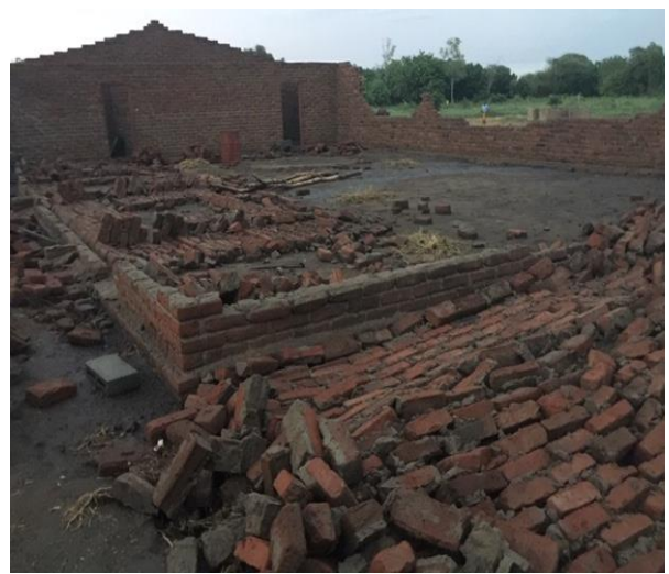
Our new church after the tornado circled inside it and blew out the walls.
