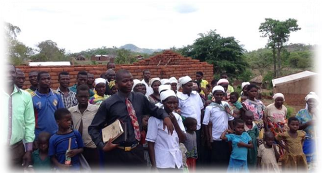
This is a church built by its congregation that needs a roof. It will cost about $500 for iron sheets.
