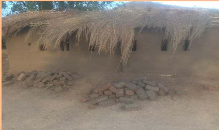
The church at Nkopola which has just been built. It needs to have the walls plastered and iron sheeting to replace the thatch.
